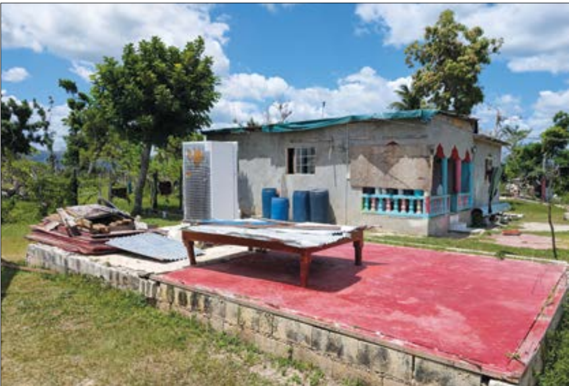
All that remains of this building is the foundation. PHOTOS COURTESY OF THE DIOCESE OF JAMAICA AND THE CAYMAN ISLANDS
